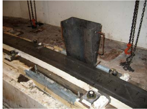
The track section alignment is verified, forms are readied for extruding cementous grout under the track and sole plates.
